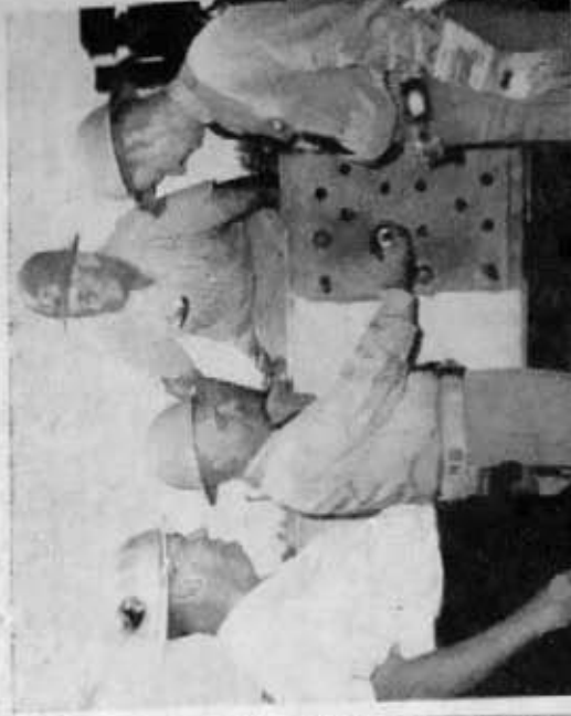
REAR ADMIRAL H. B. JONES , officer in charge of construction for the 5th Naval District, draws the first bolt into place as steel work began last Thursday on what will become the world's largest radio telescope. Looking on, from left, are T. W. Wommack, superintendent for the prime contractors, T.K.P., C. O. "Slim" Edmonds, construction superintendent for American Bridge Company, and Capt. Frank C. Tyrrell, resident officer in charge of construction for the Navy.
